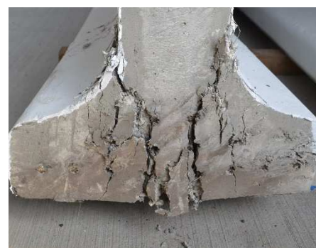
(b) strand penetration Beam 3
